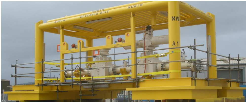
Figure 3-9 - Typical SSIV structure, analogous to that to be installed on the Teesside Pipeline
